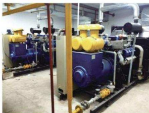
菲律宾某污水厂电站项目 A sewage treatment plant power station project in the philippines
